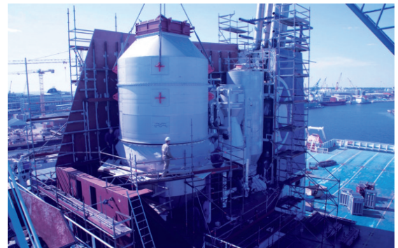
Figure 23 Scrubber retrofit 전경
